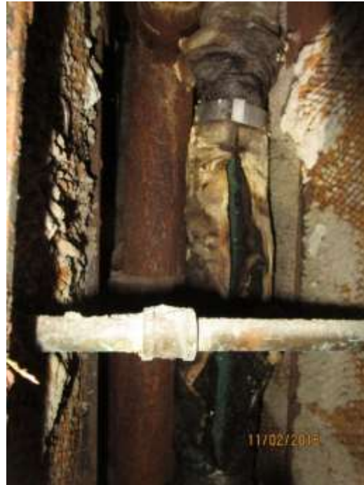
Damaged insulation on cold water riser
