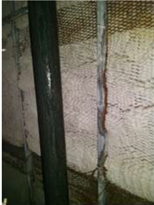
Missing insulation on cold water riser
