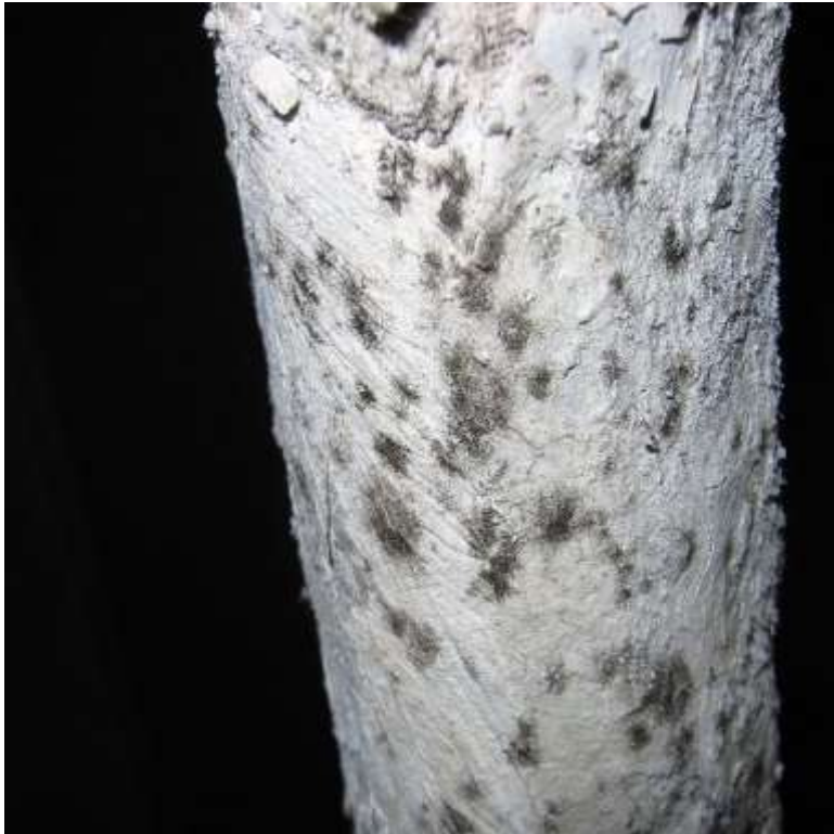
ACM- Pipe insulation (T.S.I)
