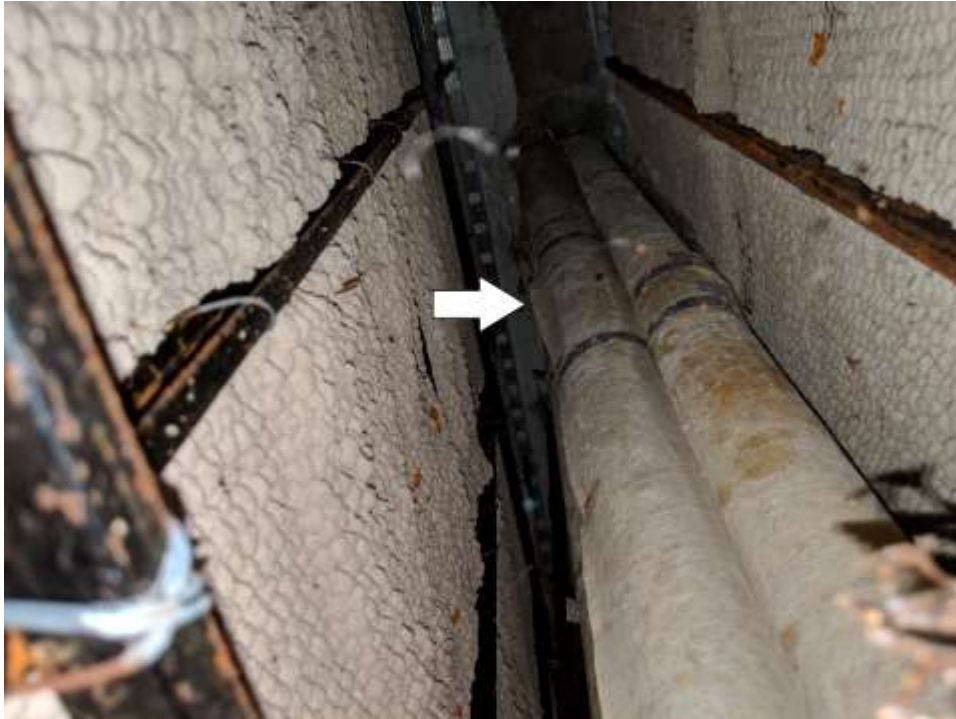
ACM- Pipe insulation (T.S.I)
