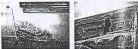
Figure 1. Walls contaminated with a thick, slimy fungus later identified as Stachybotrys .
